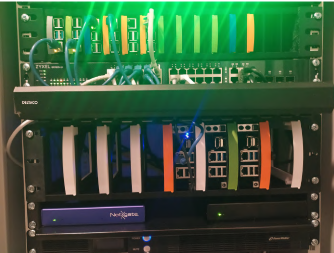
Figure 22 - The final assembly mounted into a rack, with 3 ODRROID-H2 units installed
